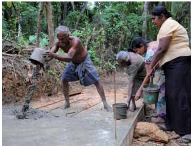
Villagers in Sri Lanka constructing an evacuation route. Community response teams developed with support from the tsunami operation CBDRR programme identified the need and the land to build the route (Daniel Cima, American Red Cross).
